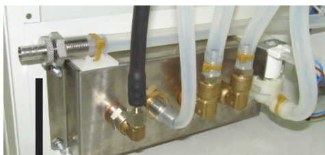
Cooling circuit valve
